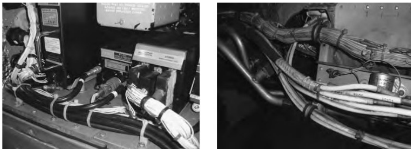
Fig. 12. Examples of installed wire looms
